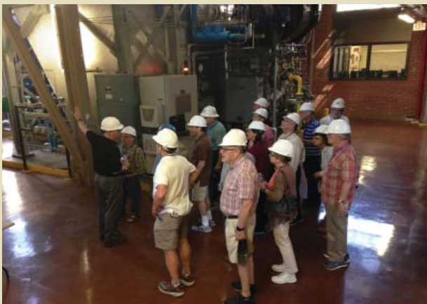
Russell Thompson and Casey Collins taught the energy class in Chilled Water Plant #2 and the West Campus Steam Plant (pictured here).
